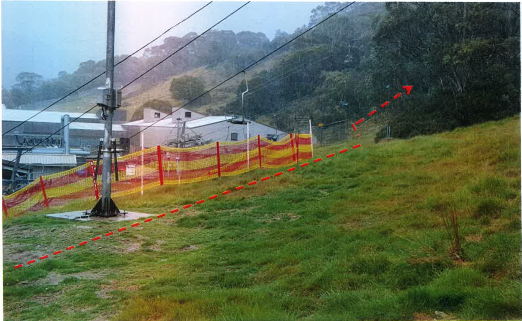
Pictures showing cable route just above Snow gum chair lift shed coming around to the old tennis courts.
